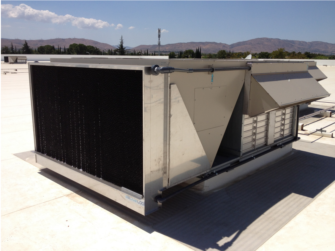
Photo and caption: “Typical DualCool® on Lennox 20 ton Rooftop Unit”
